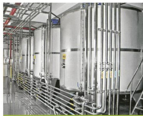
调配系统 Mixing System
